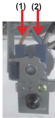
Pilot Valve Machine Room
