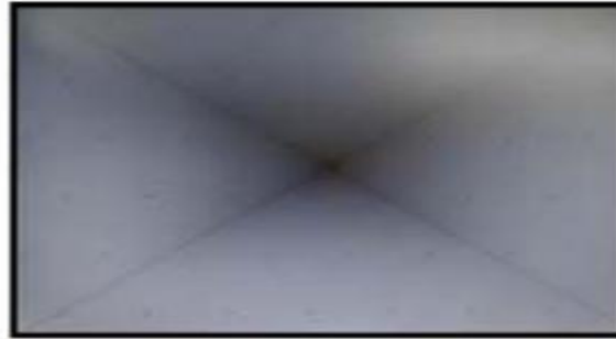
Abnormal Power Section
