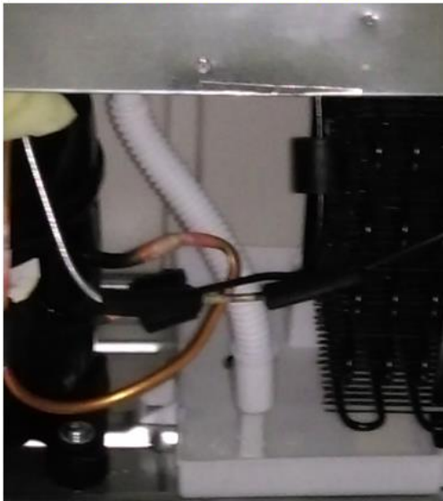
Freezer draining group
